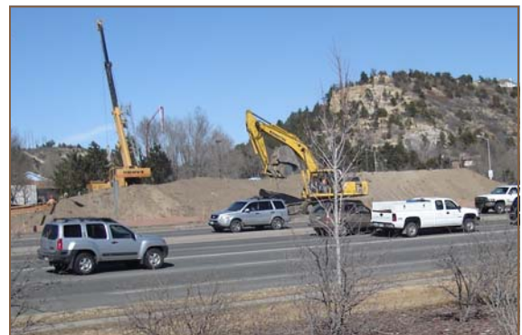
The Austin Bluffs Parkway and Union Boulevard intersection is a high accident-prone location. A major capital project is now under way to reduce these traffic concerns (see page 2).
